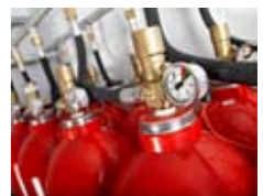
Fire Suppression Installation
